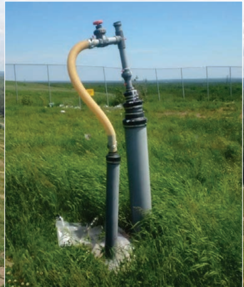
Figure 8: A completed vertical LFG Well
