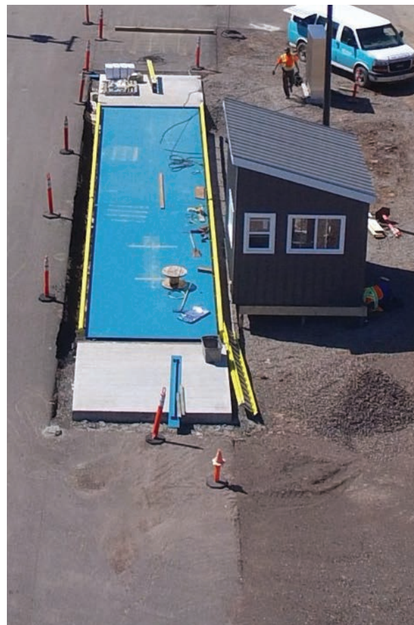
Figure 1: New Scalehouse and Weigh Scale at Public Drop Off
