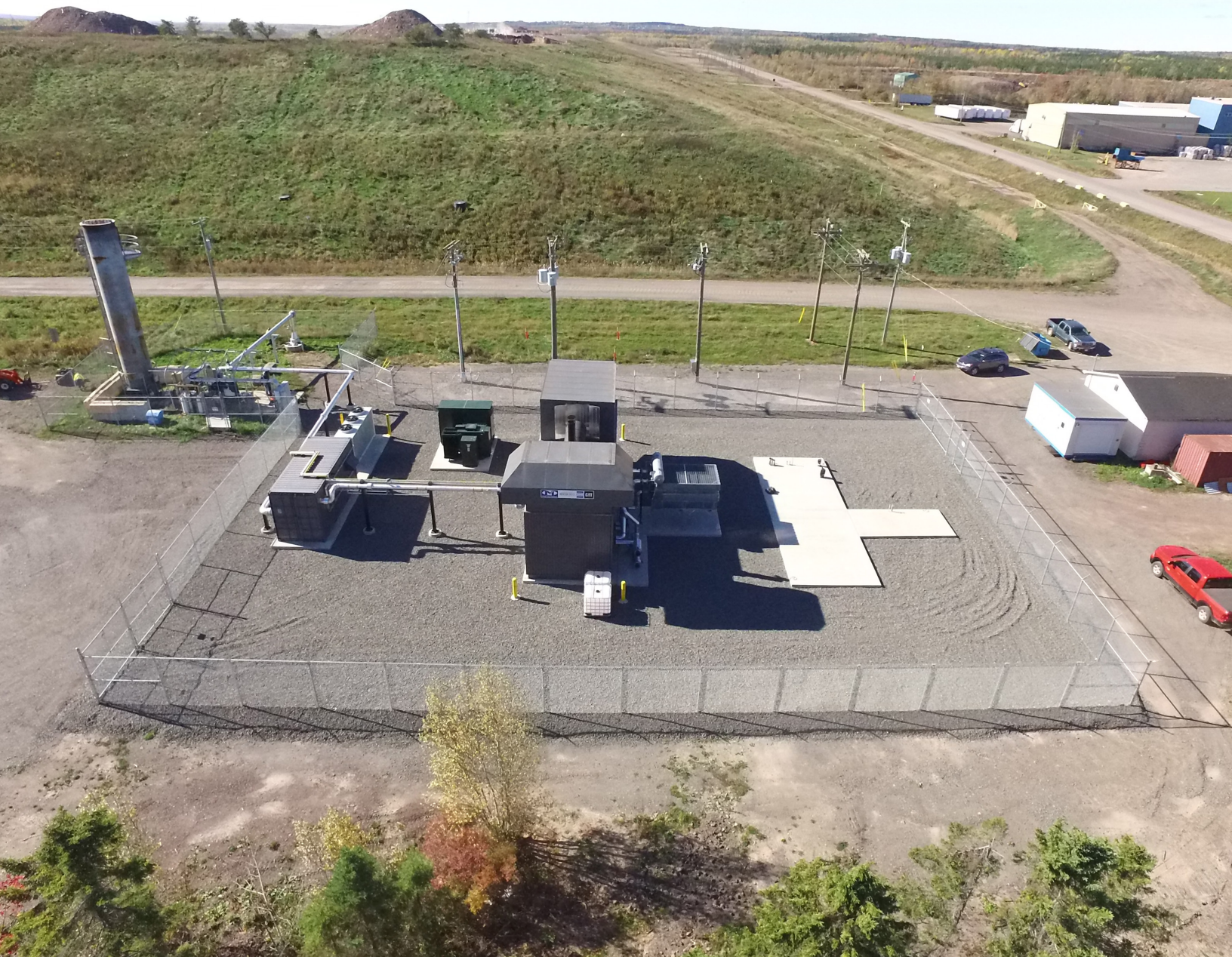
Landfill Gas-to-Energy generator and flare
