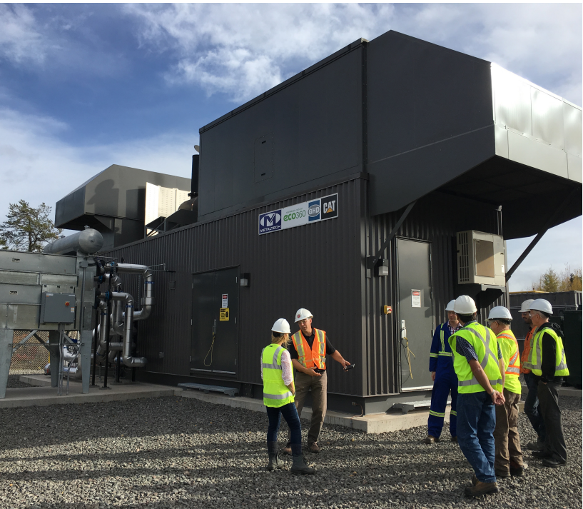
Landfill Gas-to-Energy generator outside view
